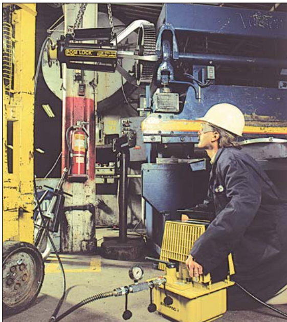
◀ An EPHR-116, 50-ton hydraulic Posi Lock® puller easily removes the main drive gear from this metal forming brake press.
